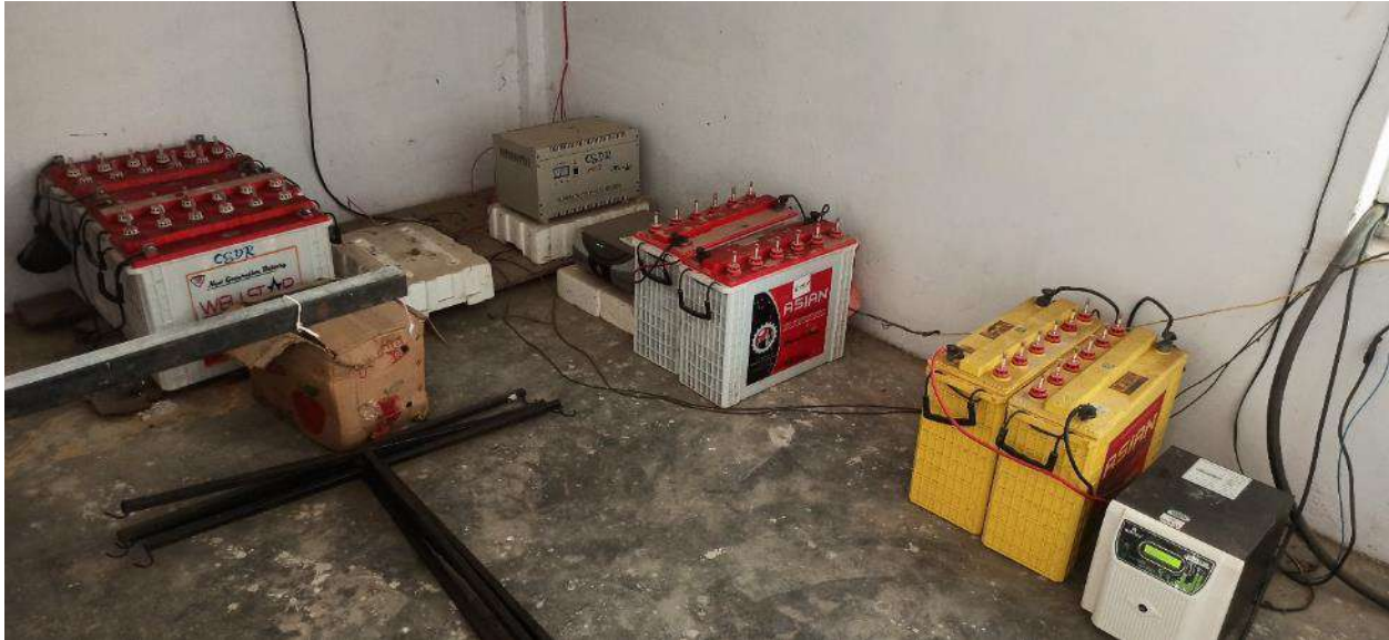
Figure 17: Battery and inverter backup in Rajapur, Bardiya
